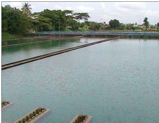
Horizontal Sedimentation Tanks, Iju Headworks.
