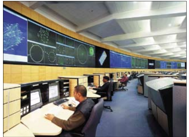
Telkom National Network Operating Center (NNOC).
